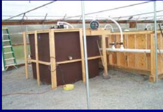
6 ft x 6 ft x 6 ft fiberglass tank
