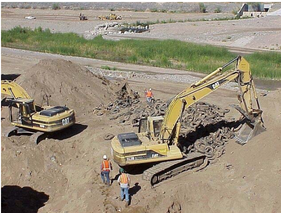
Rio Salado low-flow channel site preparation Photo courtesy of Karen Williams, City of Phoenix, Arizona
