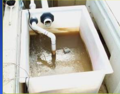
Backwash Water Sump
